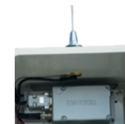
External Antenna with Surge Arrester
